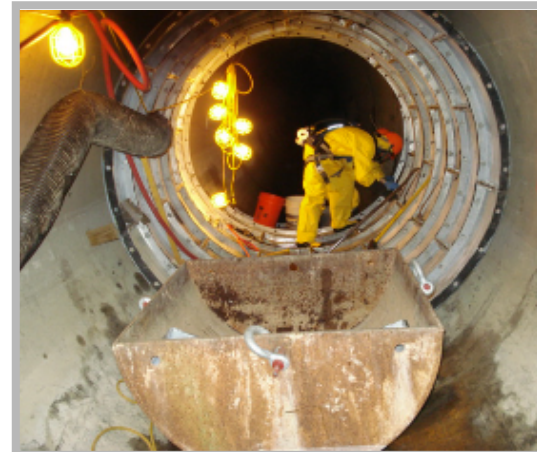
Lighting, Ventilation, and Video Monitoring
