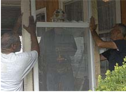
A crew installs a new window after repairing a front porch. Workers also fixed plumbing, painted rooms, repaired railings and replaced bathroom fixtures.
